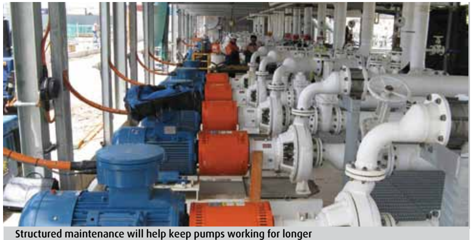
Structured maintenance will help keep pumps working for longer
