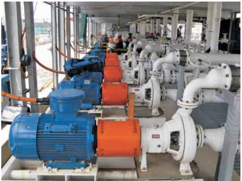
Centrifugal pumps installed at one of the largest liquid storage terminals in Australia
