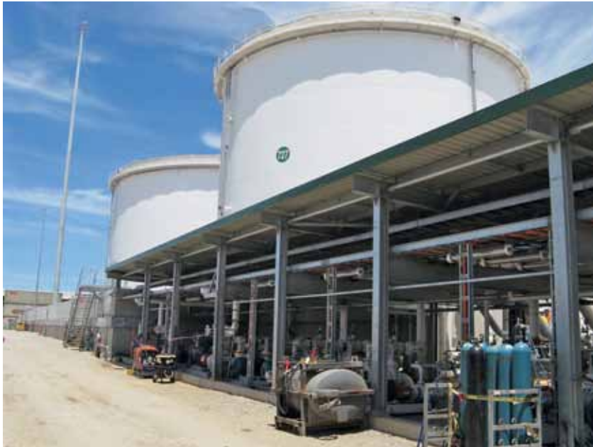
Pumps are the heart of any liquid storage terminal operation.
